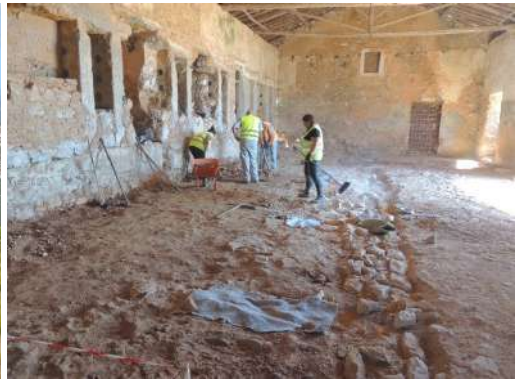
Figure 2. General view of the archaeological work carried out inside the Quinta da Serra or Retiro olive oil mill.
